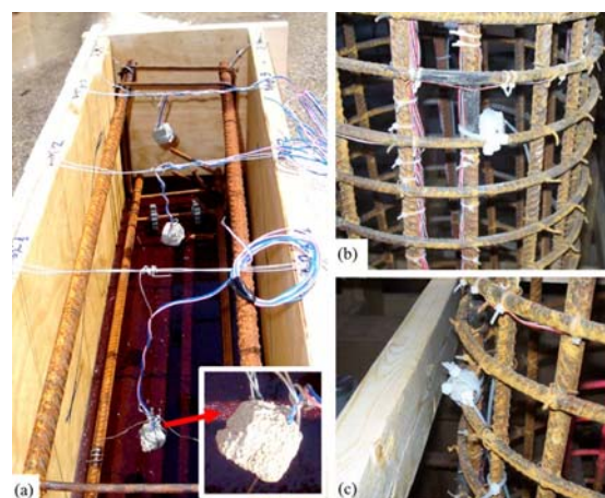
Figure 2. Fixing PZT SA inside structural elements: a) installation of PZT SA inside the wooden formwork of RC beam [2], b-c) A PZT SA fixed on the rebar cage of column [3]
