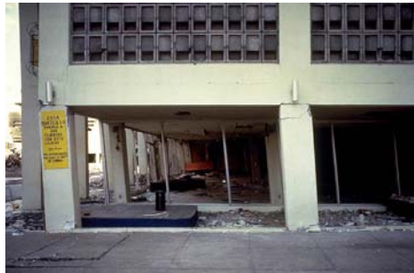
Figure 1. Soft-story mechanism in the ground floor.
